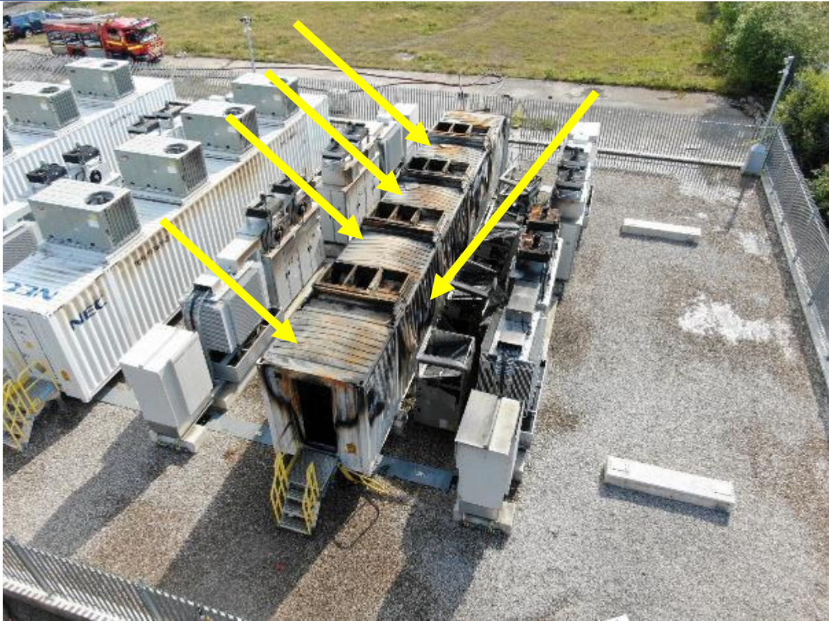
Image 2 shows the damaged container with signs of expansion/distortion that is equal across the container and not localised to the area of the initial failure.
