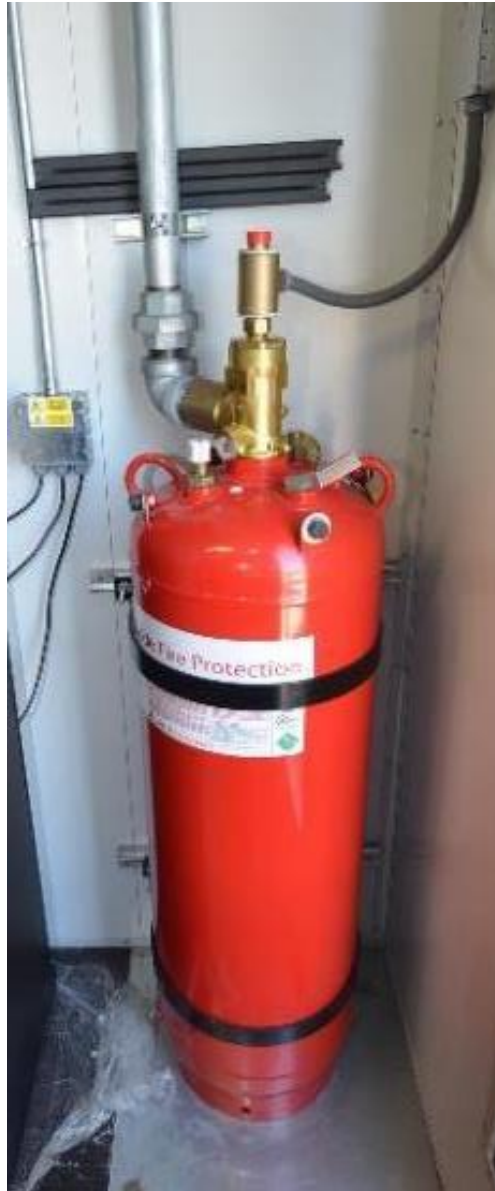
NOVEC system in unit two
