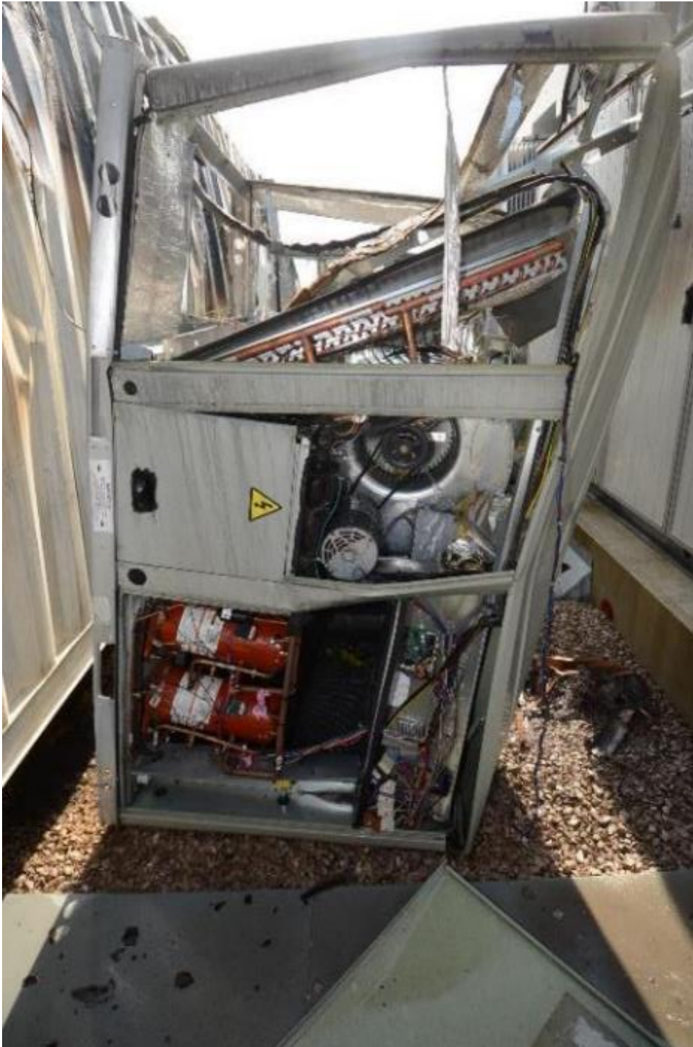
HVACS after coming dismounted from the container roof
