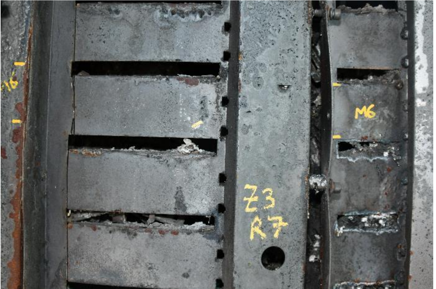
Image MB0_7397 shows where module 6 would have been pre fire. The modules had melted and collapsed.
