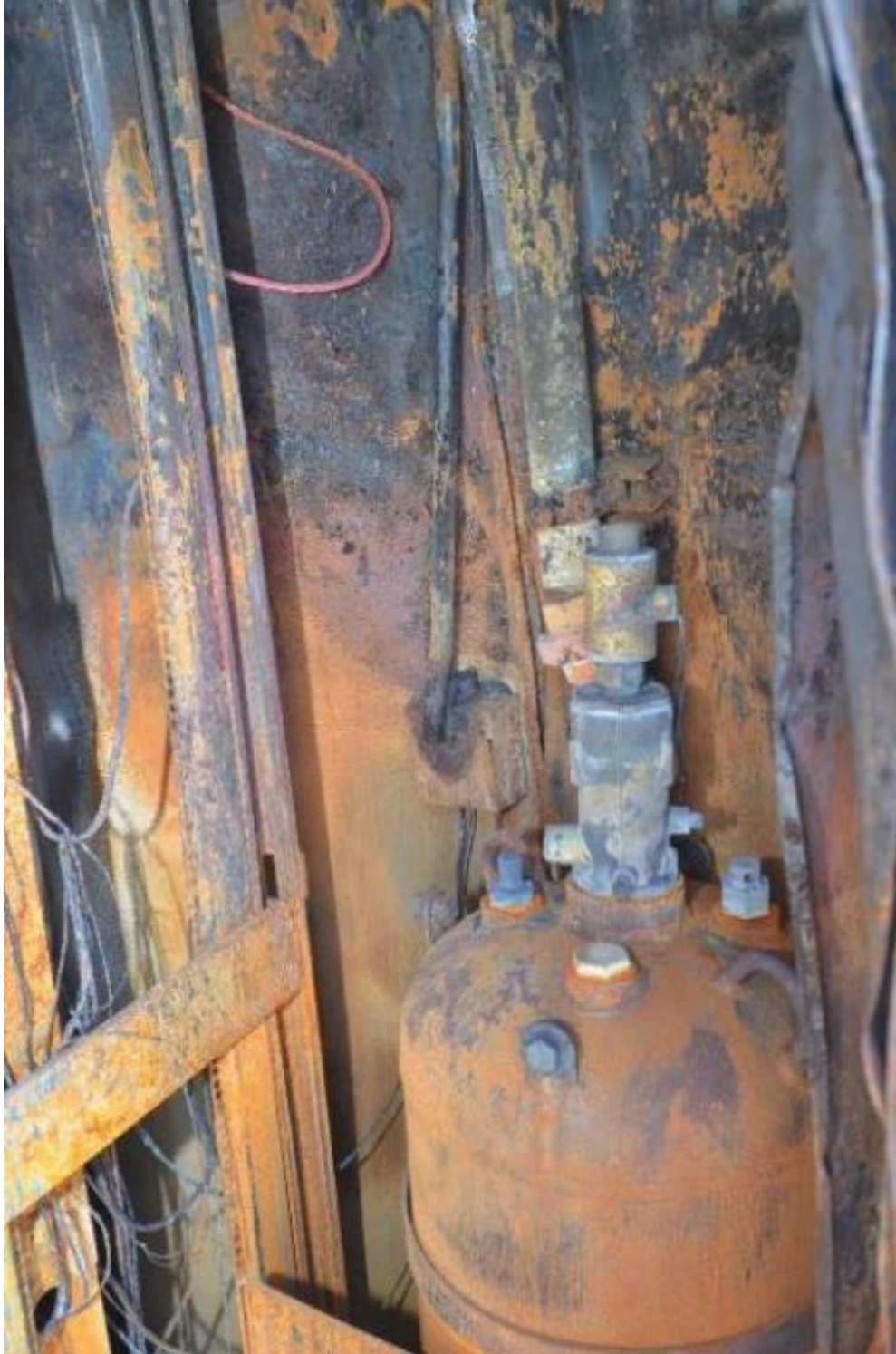
NOVEC system in container one with damaged pipe work
